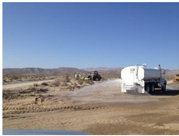
Photo 8: A water truck is utilized at the laydown yard for compaction and dust suppression.
