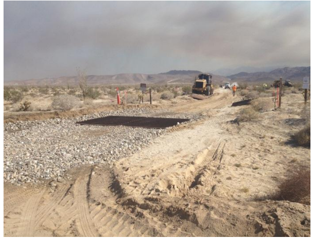
Photo 2: A rock apron and rattle plate is constructed at the primary project access point adjacent to County Route S2 and the temporary laydown yard. The rattle plate and rock apron is being utilized to minimize track-out along County Route S2.
