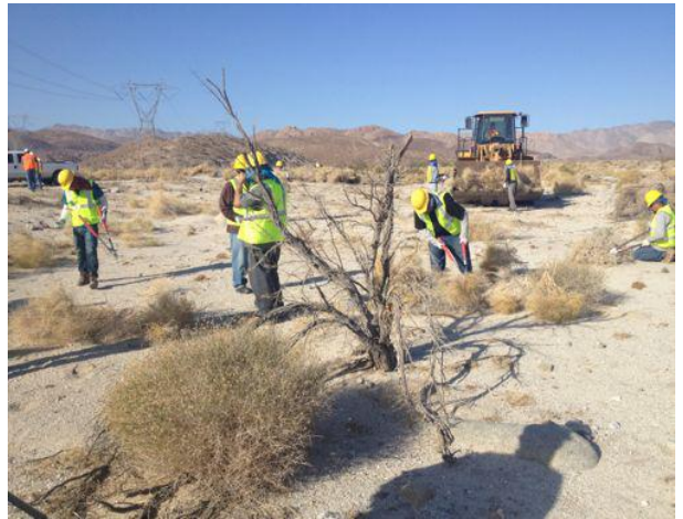
Photo 4: Hand crews clear vegetation within the approved work limits at the 30-acre substation/switchyard.
