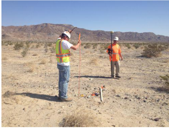
Photo 5: Surveyors placing stakes at the 30-acre substation/switchyard to identify the approved work limits.
