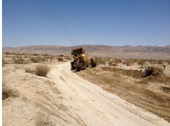
Photo 6: A road grader is utilized to construct an access road from the laydown yard located adjacent to County Route S2 and the 30-acre substation/switchyard.
