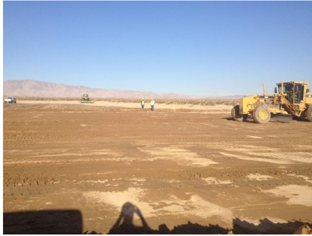
Photo 1: A road grader is utilized to construct a level pad site at the temporary laydown yard located adjacent to County Route S2.
