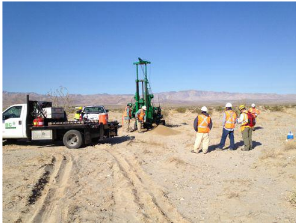
Photo 7: A geotechnical crew completes geotechnical testing at a future location for a wind turbine foundation.
