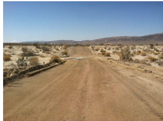
Photo 4: The access road between Dos Cabezas Road and the 30-acre substation switchyard has been completed.
