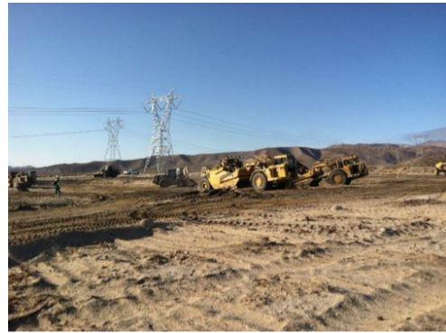
Photo 6: Heavy equipment is utilized to establish the 30-acre substation/switchyard pad site. Transmission towers associated with the Sunrise Powerlink and Southwest Powerlink can be seen in the background of this photo.
