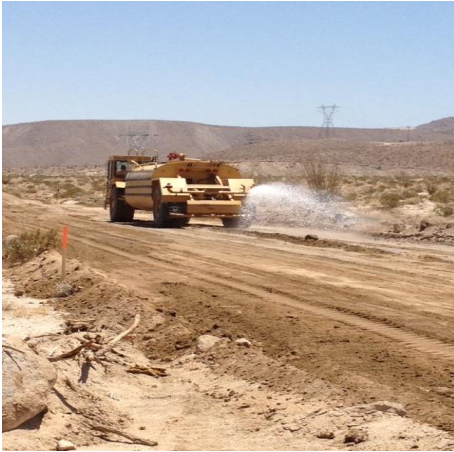
Photo 1: A water truck is utilized for dust suppression and grading compaction purposes along the access road between Dos Cabezas Road and the 30-acre substation/switchyard.
