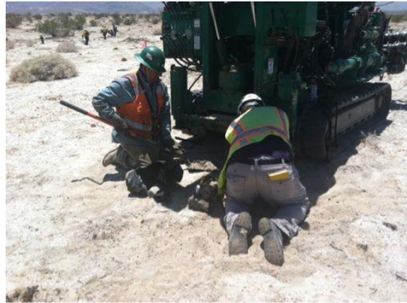
Photo 2: A crew repairs a drill rig where a hydraulic hose leak was identified. The hose was repaired and the area was cleaned up in accordance with project requirements.
