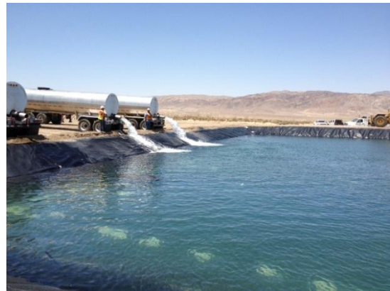
Photo 8: Water trucks placing water within the temporary water storage pond located at the temporary laydown yard.
