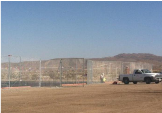
Photo 7: A 10-foot tall chainlink fence is constructed along the perimeter of the temporary water storage pond.
