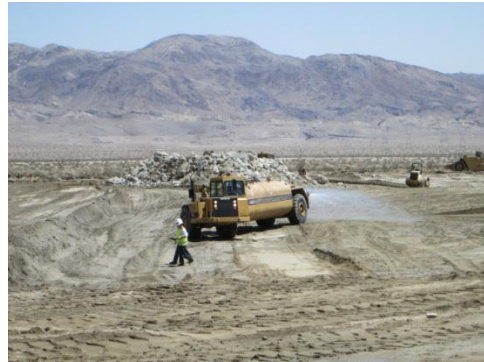
Photo 2: Active construction areas are being watered down for dust suppression purposes during grading activities at the substation/switchyard.
