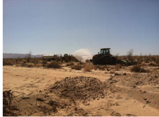
Photo 2: A water truck is utilized for dust suppression during flailing activities at the laydown yard.
