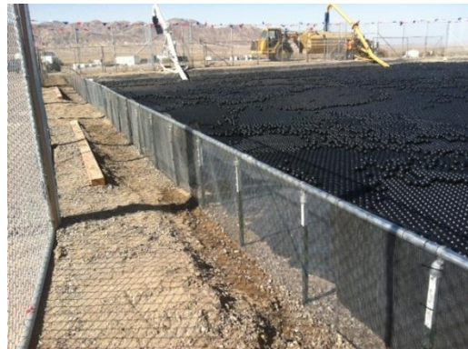
Photo 6: Armor balls have been placed along the water surface at the temporary water pond in accordance with Section 4.2 of the Raven Control Plan (MM-Wild-1j).
