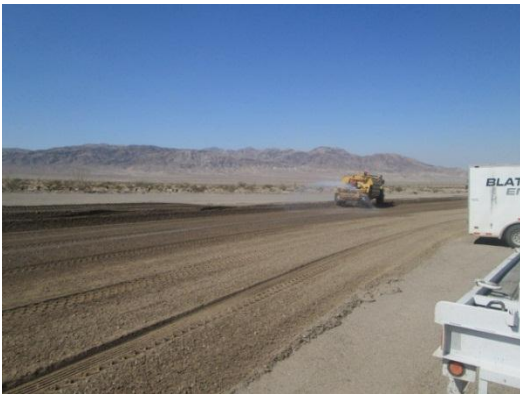
Photo 3: A water truck is utilized during grading activities associated with establishing the laydown yard.
