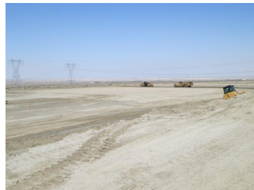
Photo 8: Crews completing grading activities at the substation/switchyard to obtain the final grade for the substation/switchyard pad site.
