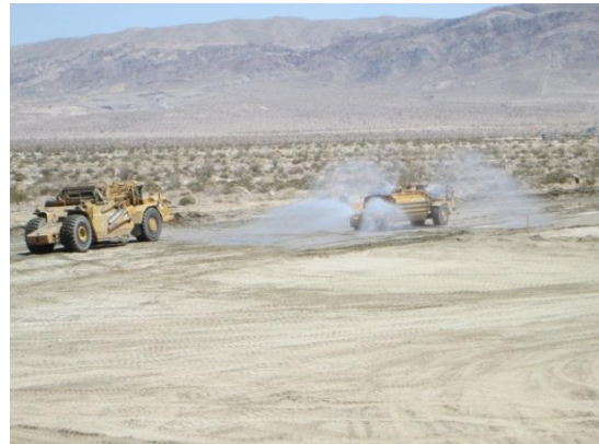
Photo 4: A water truck being utilized for compaction and dust suppression purposes at the substation/switchyard.
