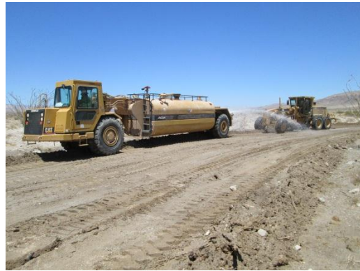
Photo 4: A water truck is utilized during grading activities associated with establishing the access road between WT 131 and WT 176.
