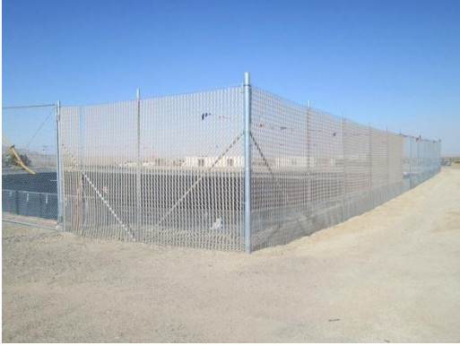
Photo 1: Fencing slats are placed along the southwestern limits of the temporary water pond to reduce the wind effects of potential armor ball movement within the temporary water pond.
