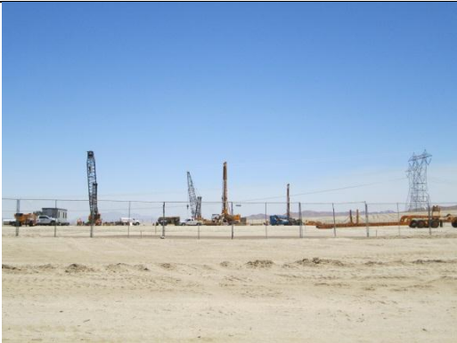
Photo 7: Crews initiated Phase II of the substation/switchyard construction by mobilizing construction equipment to the graded pad site.
