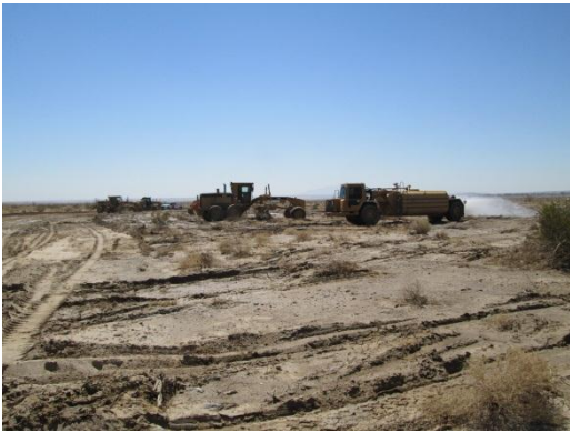
Photo 3: A water truck is utilized for dust suppression and compaction purposes associated with establishing the foundation for a wind turbine pad site.
