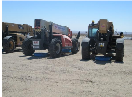
Photo 2: Drip-pans are placed beneath construction equipment staged onsite to ensure equipment does not leak directly onto the ground surface.
