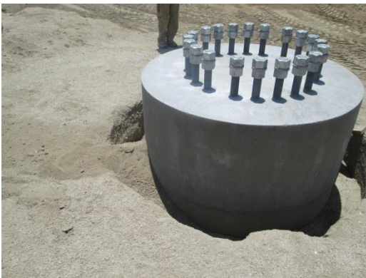
Photo 3: Wildlife escape ramps are constructed at foundations within the substation/switchyard in accordance with MM-Wild-1b.
