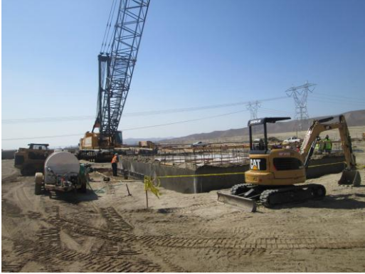
Photo 5: Crews construct foundations that will be utilized to erect above grade components associated within the SDG&E substation.
