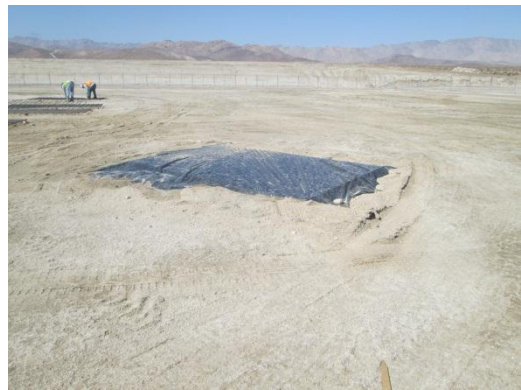
Photo 4: Covers are placed over areas excavated within the substation/switchyard in accordance with MM-Wild-1b.
