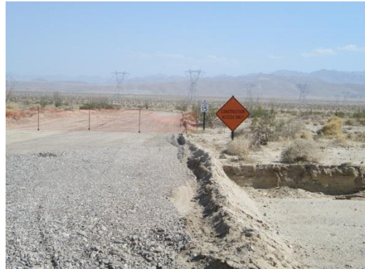
Photo 8: Signage has been placed at the point of ingress/egress to turbine string roads that intersect with public roads to notify motorists and the public that construction access is only permitted along turbine string roads for public safety purposes.
