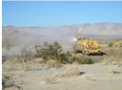
Photo 2: A water truck applies water during grading activities to minimize dust emissions in accordance with the Dust Control Plan.
