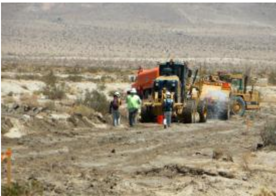
Photo 3: Archeological and Native American monitors complete monitoring activities during ground disturbance activities associated with establishing the access road along Dos Cabezas Road.
