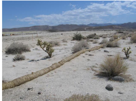
Photo 12: Straw wattles are repaired in areas that were damaged during the rain event on 7.13.12.
