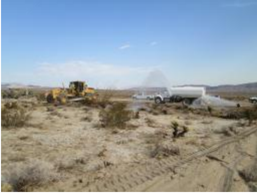
Photo 5: Crews complete grading and clearing activities at WT 149. A biologist, archeologist and Native American monitor are present during grading activities per the project requirements.
