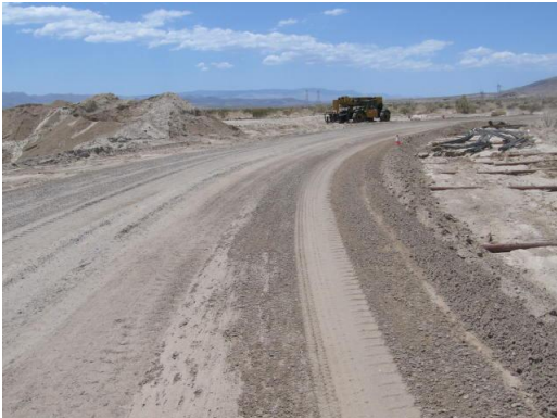
Photo 11: Construction crews repair access roads following the rain event that occurred on 7.13.12.
