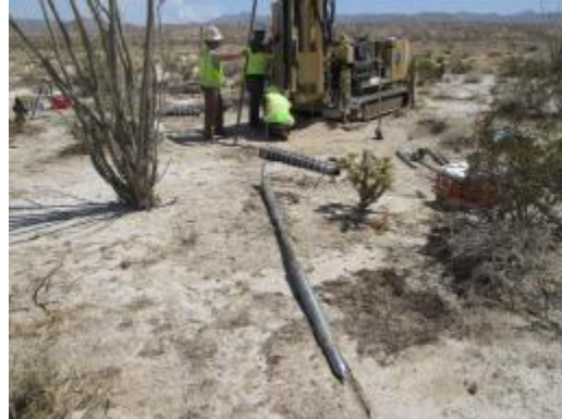
Photo 8: A geotechnical rig completes geotechnical testing activities within the approved work limits at Wind Turbine 50.
