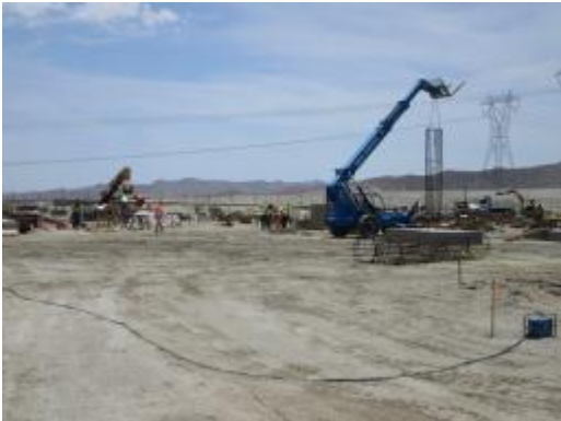
Photo 7: Crews place steel rebar within an excavation for the foundations that will be utilized to construct substation components.
