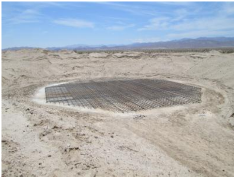
Photo 7: A concrete foundation with steel rebar is constructed at the wind turbine pad base that will be utilized for the construction of a wind turbine.
