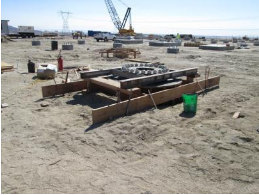
Photo 5: A foundation is constructed within the SDG&E substation that will be utilized to transfer energy generated from the wind turbines to the Sunrise Powerlink located along the eastern limits of the substation.
