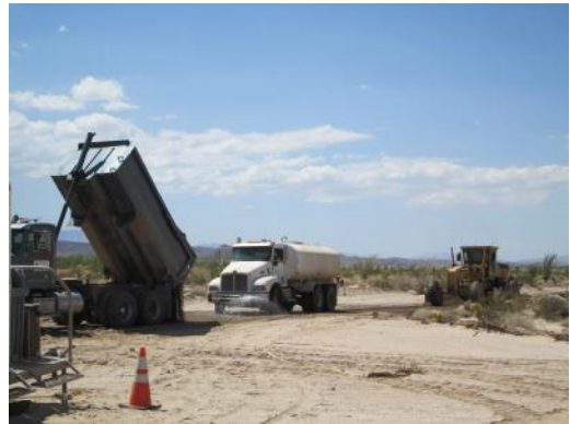
Photo 8: Gravel road base is placed along turbine access roads. A water truck is utilized to suppress dust during placement of the gravel road base
