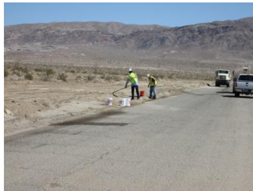
Photo 4: A crew cleans a hydraulic leak with a spill kit in accordance with the project requirements.
