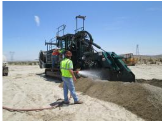
Photo 8: A track trencher is utilized to place the 34.5 kV collection lines underground within the approved work limits.
