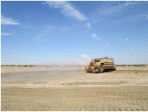
Photo 1: A water wagon is utilized to pre-water a wind turbine foundation pad prior to excavation activities to minimize dust emissions in accordance with the Dust Control Plan (MM-AIR-1).
