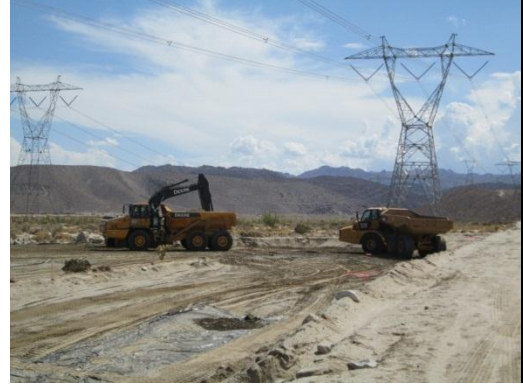
Photo 6: Construction crews were observed creating a pad site for the turning structures that will be used to deliver power generated from the wind turbines via the Substation/Switchyard to the Sunrise Powerlink
