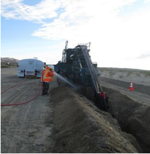
Photo 1: Construction crews utilize water to minimize dust emissions during trenching activities for installation of the 34.5 kV underground collection lines in accordance with the Dust Control Plan (MM-Air-1).
