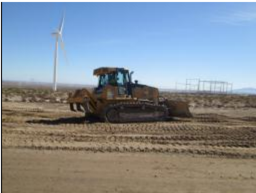
Photo 7: Crews backfill along the collection line corridors following the installation of 34.5 kV collection lines that will be utilized to deliver power from the wind turbines to the onsite substation.
