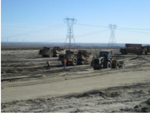
Photo 5: Biological monitors are present during ground disturbance activities to ensure all activities are completed within the approved work limits per MM-Wild-1d.
