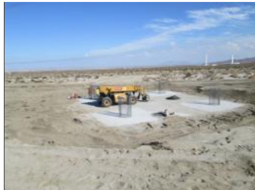
Photo 8: Construction activities continued during this reporting to establish the concrete foundations for the Sunrise Powerlink turning structures.
