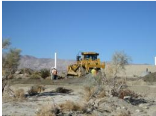
Photo 1: Archeological monitors complete monitoring of initial ground disturbance per the project requirements.
