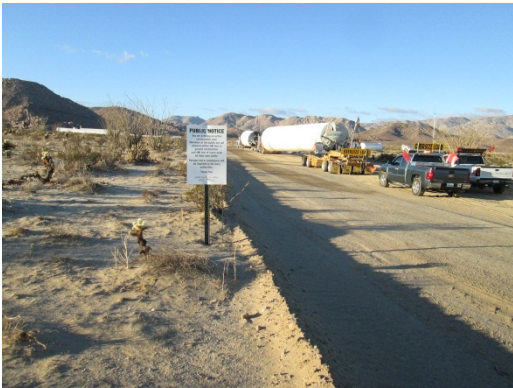
Photo 7: Turbine part deliveries and mobilization continued during this reporting period. Delivery trucks utilized clearly signed access roads within the approved work limits.
