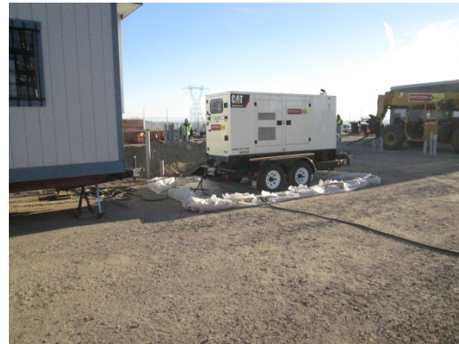
Photo 8: Secondary containment is utilized to prevent soil contamination per the SWPPP and MM-WATER 10.
