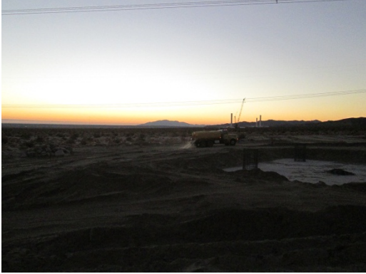
Photo 5: Water was applied before, during, and after construction activities, including the Sunrise Powerlink turning structures to suppress potential fugitive dust per MM-Air-1.
