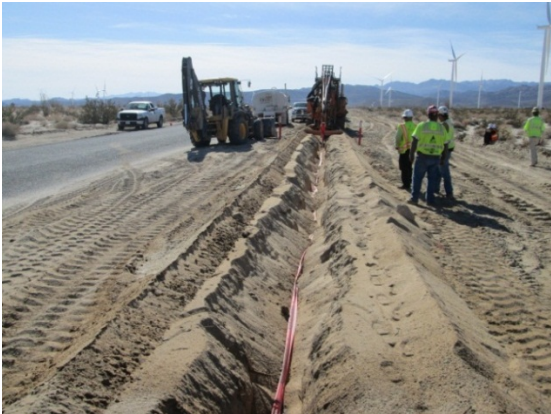
Photo 3: Biological, Archaeological, and Native American Monitors observe work along the collection line trench area situated along Mine Road
