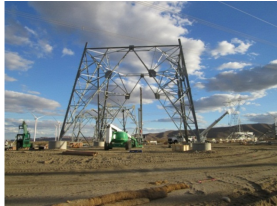
Photo 4: A lattice tower is assembled on site which will provide a connection to the South West Power Link 500kV transmission line.
