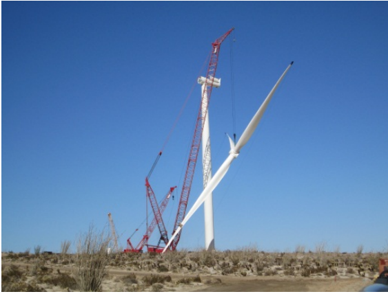
Photo 1: Turbine and Rotor Assembly is completed via use of a large crane.
