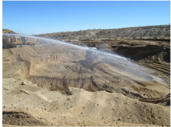
Photo 2: Turbine excavation activities are watered down to prevent fugitive dust in accordance with MM-Air 1.
