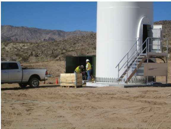
Photo 3: Electrical work associated with connecting wind turbines to the underground collector cable network continued during this reporting period.
