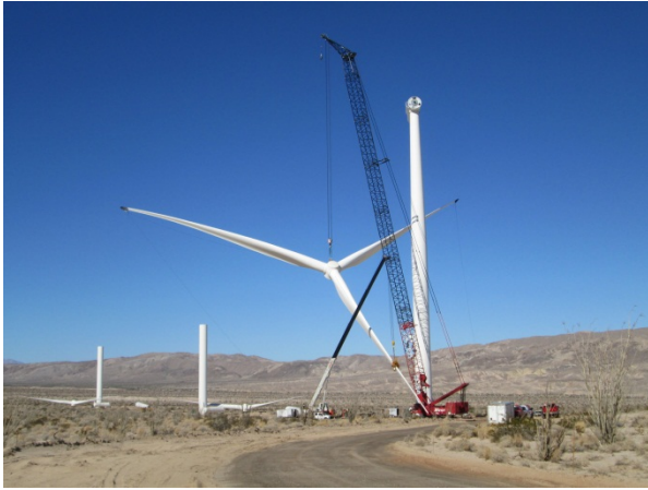
Photo 1: A large crane is utilized to assemble the rotor and blades to the nacelle at a wind turbine pad site. Ten turbines were erected this reporting period.
