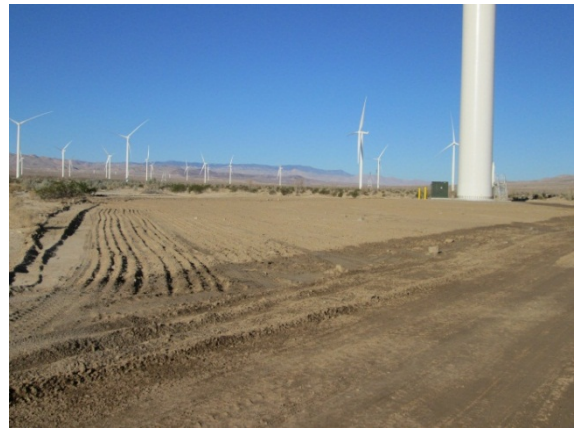
Photo 4: Topsoil staged onsite from initial ground disturbance is utilized to reclaim a wind turbine pad site in accordance with MM-Veg 2b.
