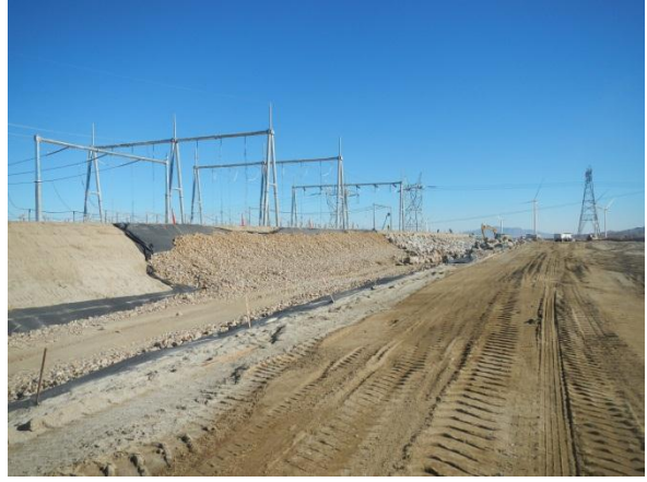
Photo 6: ECMs observed crews installing rip-rap around the substation switchyard for flood protection.
