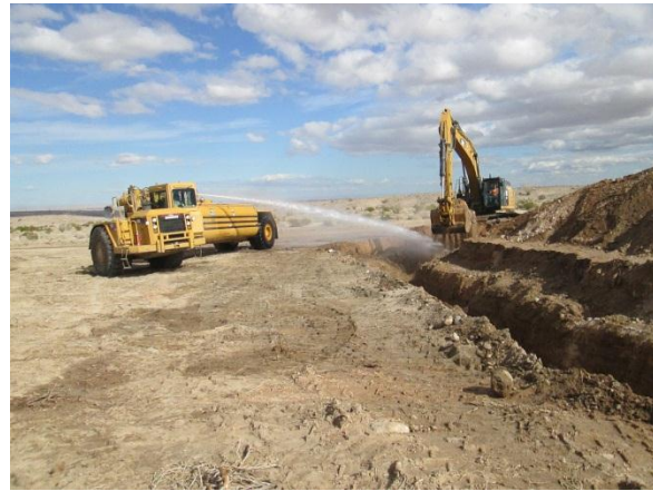
Photo 4: A water tender is observed suppressing fugitive dust during wind turbine foundation excavations in accordance with the Dust Control Plan (Mitigation Measure Air-1).
