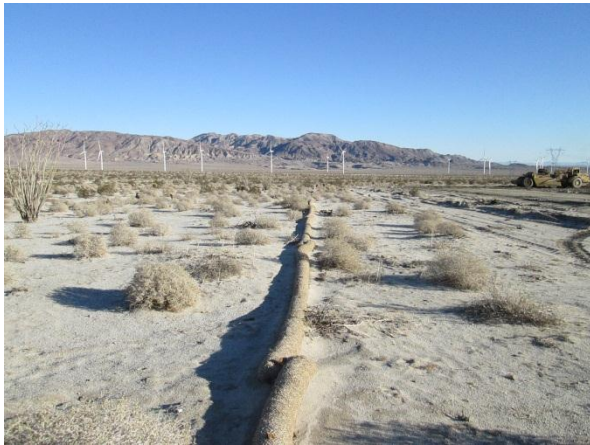
Photo 3: Straw wattles are installed along the perimeter of the Phase II Substation Grading in accordance with the SWPPP (MM WATER-9)
