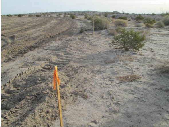
Photo 1: ECMs observed resolution of soil berms noted outside of the work limits in Weekly Report #34.
