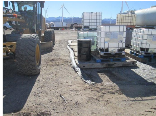
Photo 4: Hazardous materials at the laydown yard are placed within secondary containment in accordance with the SWPPP (MM WATER-9).
