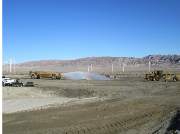
Photo 2: Water trucks apply water to the Phase II Substation grading areas in accordance with the Fugitive Dust Control Plan (MM Air-1).
