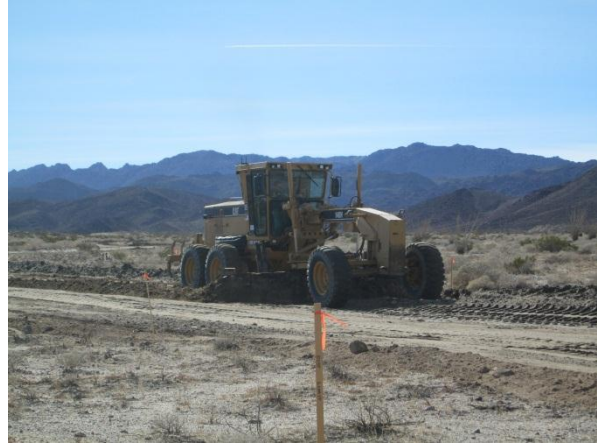
Photo 2: ECMs observed access road subgrade activities south of Interstate 8, being performed within the approved staked work limits.
