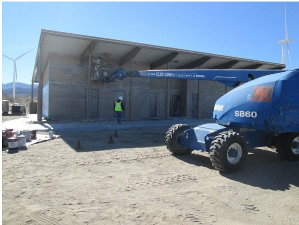
Photo 3: ECMs observed crews painting the O&M facility. In accordance with the Surface Treatment Plan (VR-3), the exterior of the facility will be painted “buff” for masonry and “brush brown” for structural steel to blend with the surrounding landscape.
