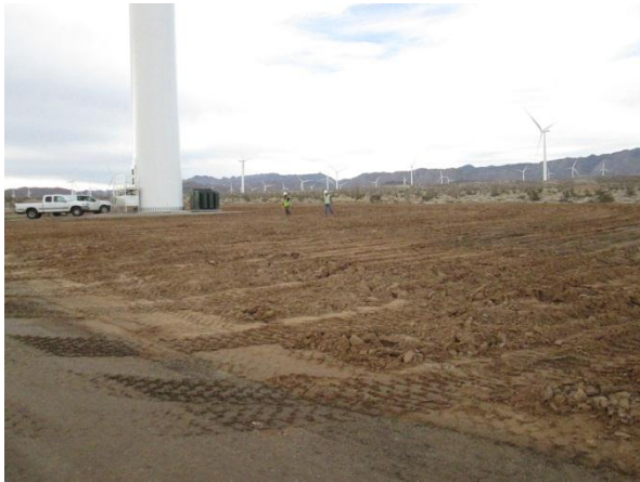
Photo 3: ECMs observed biologists measuring soil de-compaction to ensure measures identified in the Habitat Re-vegetation plan were being implemented (MM Veg-2b).
