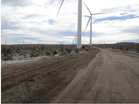
Photo 1: Reclamation of access road and collection lines occurred within with work limits as identified by staked areas.
