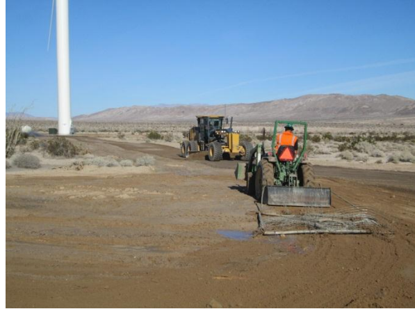
Photo 2: ECM's continued to observe reclamation activities (raking) associated with post-construction disturbance areas.
