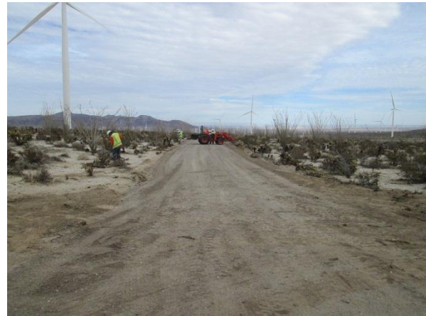
Photo 4: ECMs observed crews implementing vertical mulching and re-planting cacti in accordance with MM Veg-2b.
