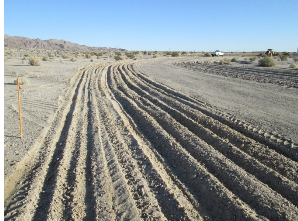
Photo 2: ECM's continued to observe reclamation activities such as soil de-compaction associated with post-construction disturbance areas within the clearly staked work limits.
