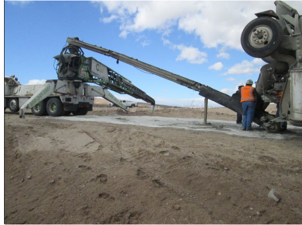
Photo 2: ECM's observed plastic being placed beneath concrete equipment in accordance with the best management practices identified in the SWPPP.
