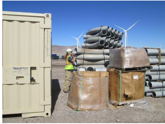
Photo 2: ECM's observed biological monitors inspecting construction piping greater than three inches in diameter in accordance with MM-Wild-1m.
