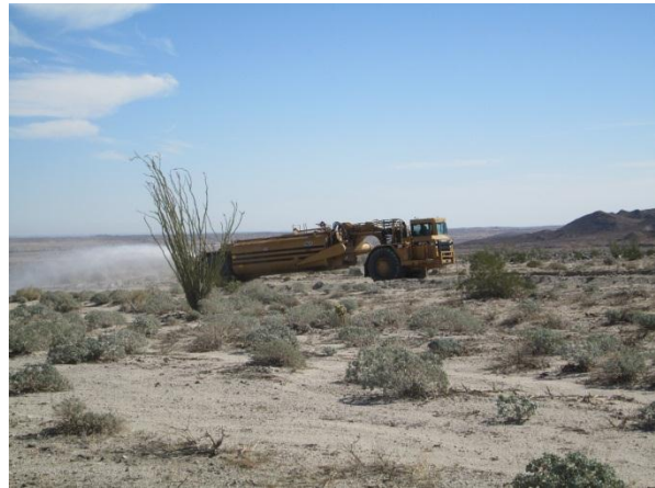
Photo 4: ECM's continued to observe access roads watered to reduce potential for fugitive dust in accordance with MM Air-1.
