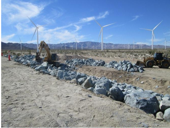
Photo 1: ECMS observed construction crews placing rip-rap around the substation for flood protection.
