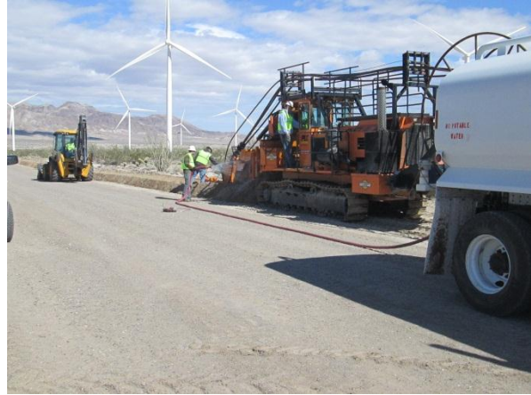
Photo 2: The placement of underground collection lines within the approved limits of disturbance continued during this reporting period.
