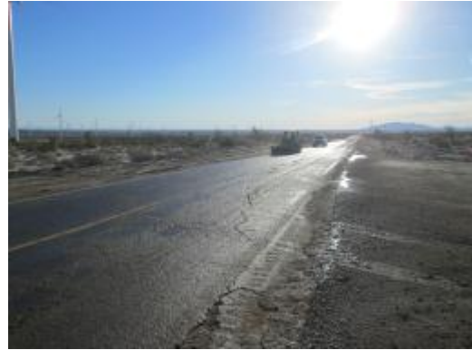
Photo 2: Highway S-2 is swept with a mechanical sweeper on a regular basis to minimize trac-out along the paved Highway in accordance with MM-Air-1.
