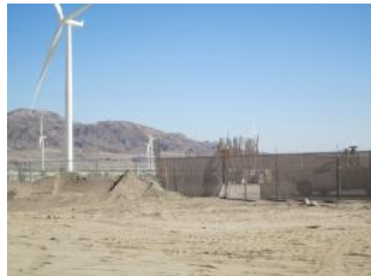
Photo 4: Crews place desert tan colored slats along the perimeter of the laydown yard associated with the O&M facility in accordance with the O&M Screening Plan (MM-VR-4).
