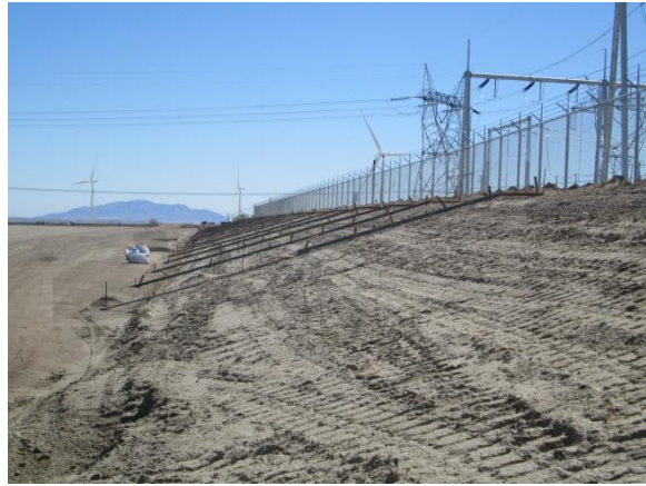
Photo 4: Work activities continue for the Phase II berm and associated flood control measures. Crews were observed utilizing shotcrete to secure slopes associated with the substation berm.
