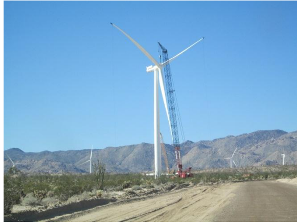
Photo 2: Turbine erection activities continued throughout the reporting period. Construction crews utilize large cranes to lift the rotor and blade for assembly with the nacelle.
