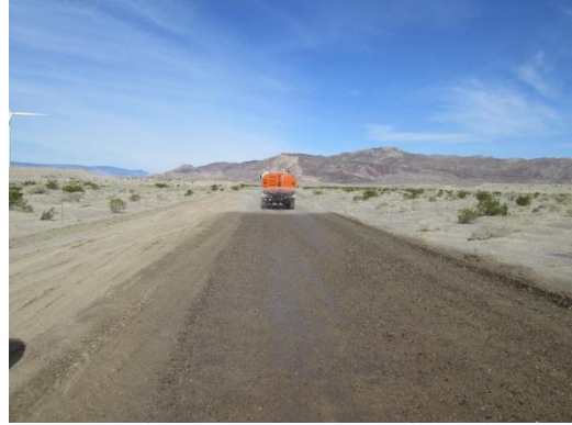
Photo 8: Water trucks are utilized to water down access roads during construction in accordance with MM-Air-1.
