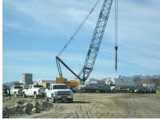
Photo 2: Turbine deliveries continued throughout the reporting period. Construction crews utilize large cranes to unload turbine components from truck trailers.
