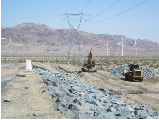
Photo 1: Construction activities continued during this reporting period associated with the berm along the perimeter of the Phase II substation.
