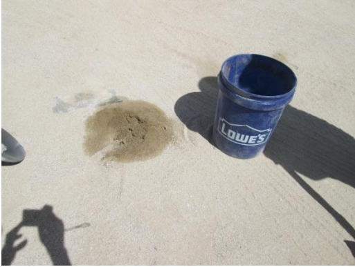
Photo 7: Crews utilize spill kits to remove stained soils in accordance with MM-Water-10.
