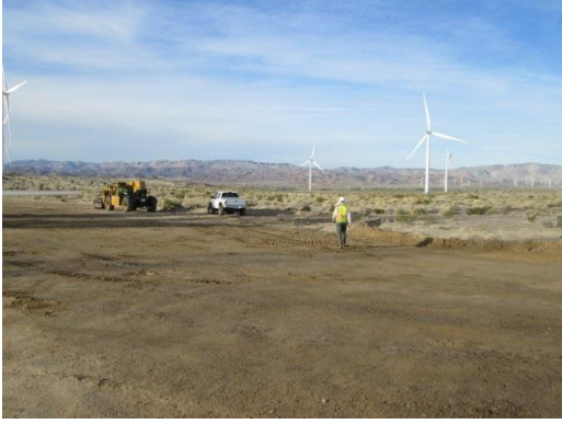
Photo 5: A FTHL permitted biologist conducts sweeps of construction areas in accordance with MM-Wild-1g.
