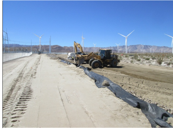
Photo 2: Construction activities associated with the berm along the perimeter of the Phase II substation continued during this reporting period.
