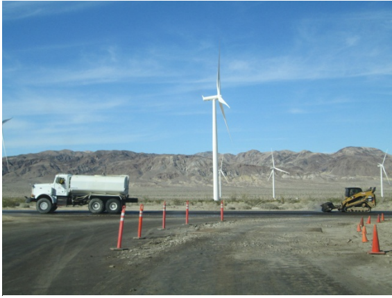
Photo 1: Construction crews sweep CA-98 to remove all debris and place cones along the project site entrance/exit to ensure that vehicles exiting the project site travel over the rumble plates and rock apron in accordance with the Dust Control Plan (MM-Air-1).
