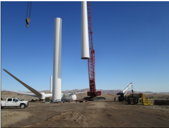
Photo 3: Construction crews utilize large cranes to lift the mid-section of the turbine tower for assembly to the base for the phase II turbines in the southeast portion of the project site.
