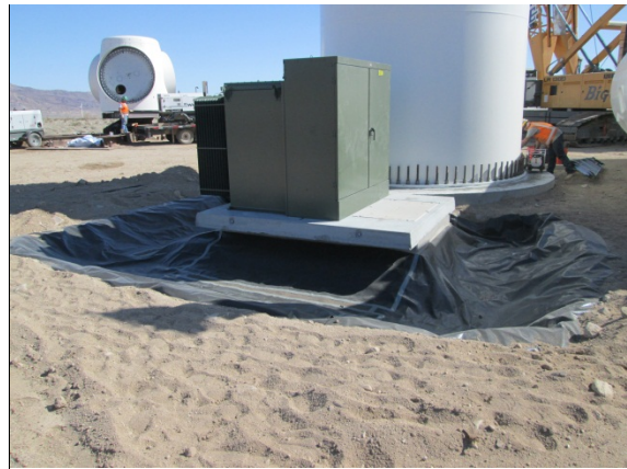
Photo 4: ECM's observed the placement of secondary containment around the perimeter of the transformer at each wind turbine pad site in accordance with the SWPPP.
