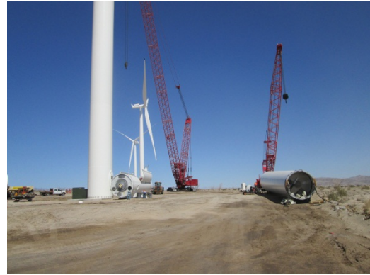
Photo 6: Large cranes are utilized to erect wind turbines associated with Phase II.
