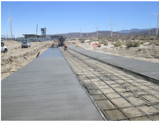
Photo 7: Work activities continued during this reporting period associated with constructing low water crossings along Dos Cabezas Road.
