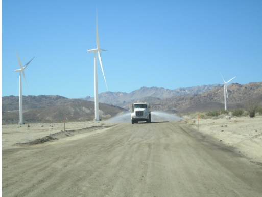
Photo 1: Construction crews water down access roads during construction activities in accordance with the Dust Control Plan (MM-Air-1).
