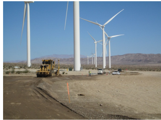
Photo 8: Grading activities being completed along the access road from Highway S-2 to the Substation/Switchyard in preparation for paving.
