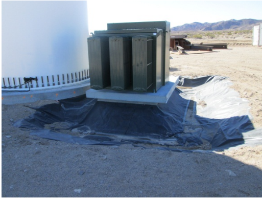
Photo 5: A secondary containment area is constructed around the perimeter of transformers located adjacent to wind turbines.
