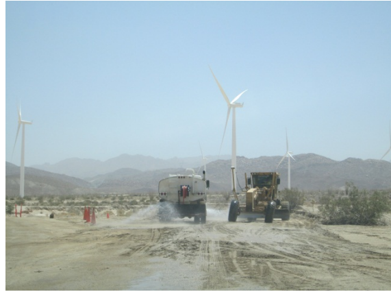
Photo 2: Water trucks are observed preventing fugitive dust as construction crews continue to construct low water crossings along Dos Cabezas Road.
