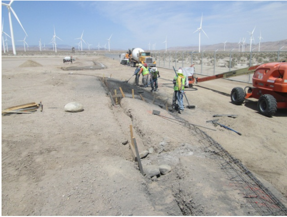
Photo 1: Construction activities associated with the berm along the perimeter of the substation continued during this reporting period.
