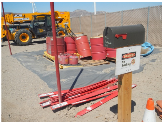
Photo 7: A "no smoking" sign is placed adjacent to the storage/refueling areas at the Laydown Yard in accordance with the Construction Fire Safety Plan (MM-Fire-1).
