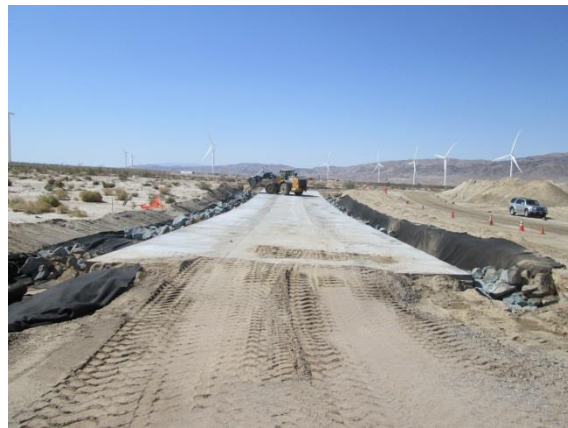
Photo 8: Work activities continued during this reporting period associated with constructing low water crossings along Dos Cabezas Road.
