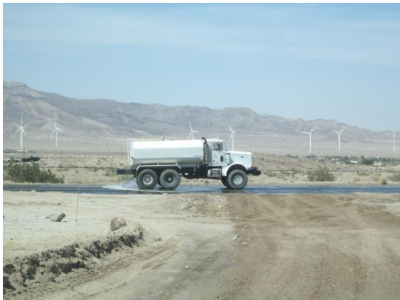
Photo 3: Construction crews clean Highway 98 to minimize track-out in accordance with the Dust Control Plan (MM-Air-1).
