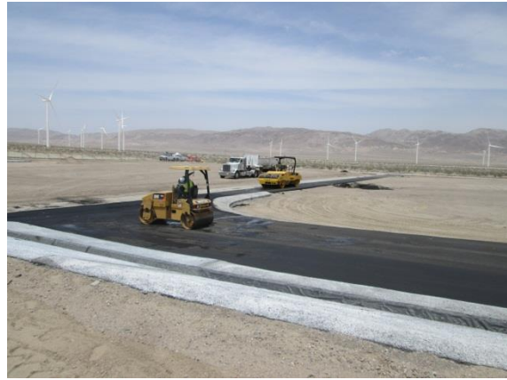
Photo 2: Construction crews were observed paving an access road within the Phase II Substation/Switchyard.
