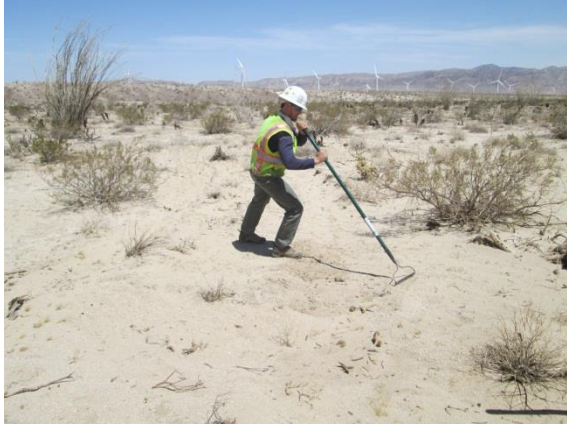
Photo 5: Construction crews use a rake to re-contour the tire tracks from tag line work in accordance with conditions of Variance Request #5.
