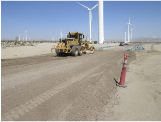
Photo 1: Crews were observed preparing the road base along Dos Cabezas Road for placement of asphalt pavement.
