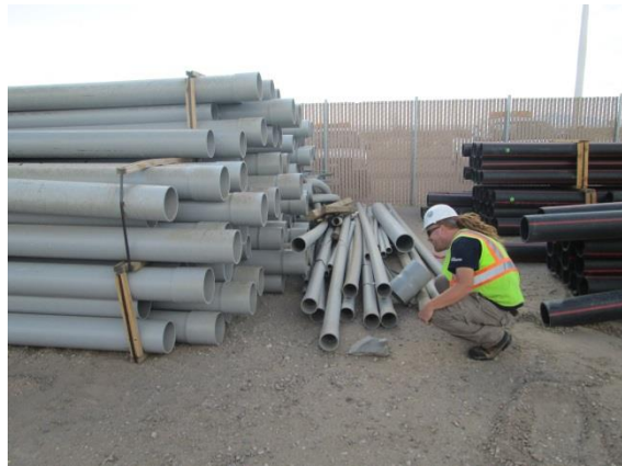
Photo 4: ECM's observed biological monitors inspecting construction piping greater than three inches in diameter in accordance with MM-Wild-1m.
