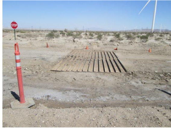
Photo 6: Rumble plates are observed to be clean and free from debris in order to minimize vehicle track-out in accordance with the Dust Control Plan (MM-AIR-1)
