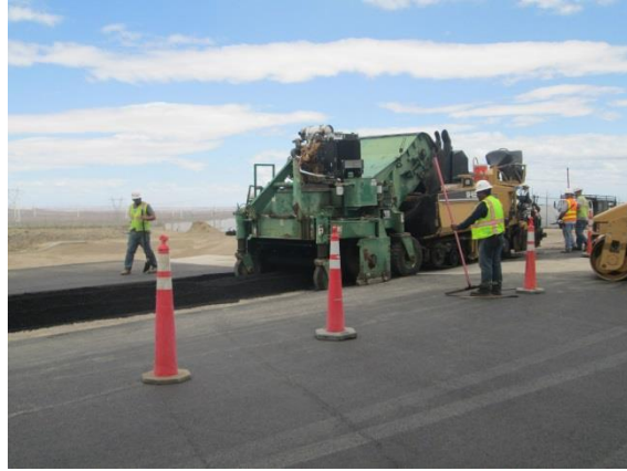
Photo 2: Construction crews paved the access road from Highway S-2 to the Substation/Switchyard during this reporting period.
