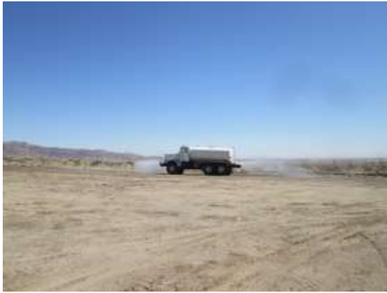
Photo 5: Construction crews water down access roads to prevent fugitive dust in accordance with the Dust Control Plan (MM-Air-1).
