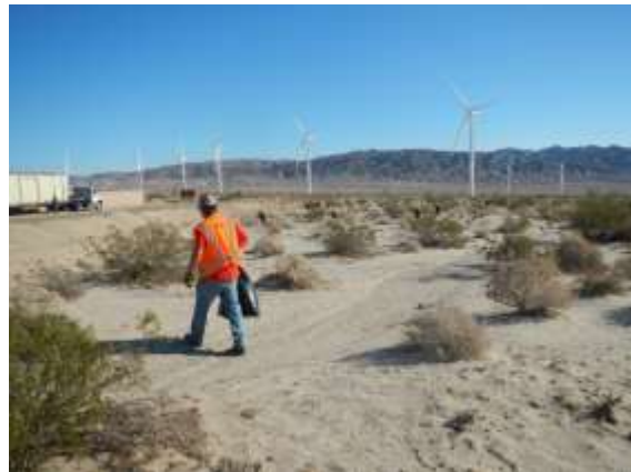
Photo 4: ECMs observed a construction crew member picking up trash in accordance with the Raven Control Plan (MM-Wild-1j).
