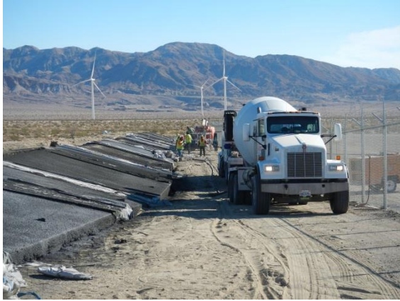
Photo 1: Construction activities associated with the berm along the perimeter of the Phase II substation continued during this reporting period.
