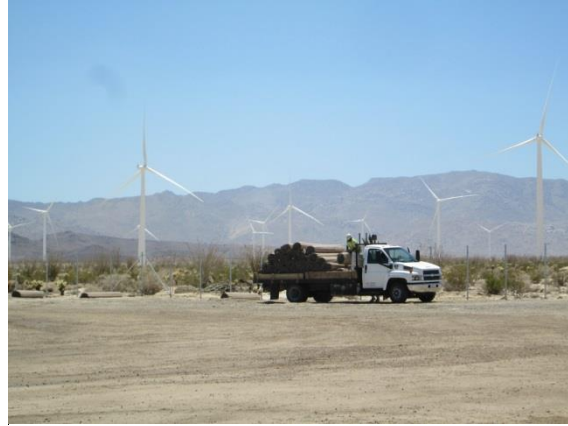
Photo 2: Construction crews began to remove the exterior Laydown Yard fence as part of the demobilization efforts.
