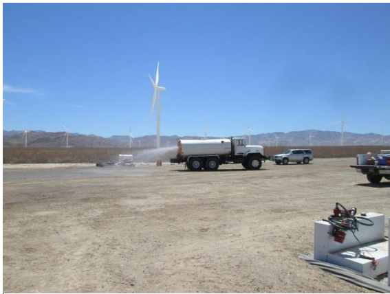
Photo 7: Construction crews water down the Laydown Yard to prevent fugitive dust in accordance with the Dust Control Plan (MM-Air-1).
