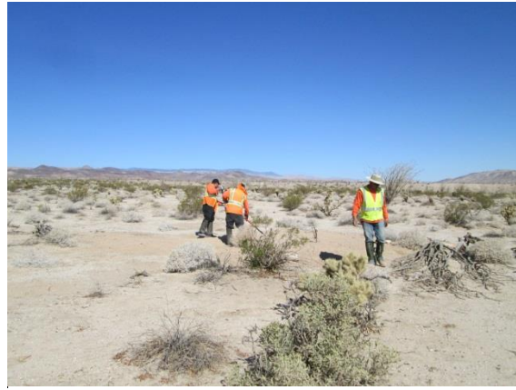
Photo 6: Construction crews use rakes to re-contour equipment tracks from the installation of artificial burrows in accordance with MM-Veg-2b and the HRRP.
