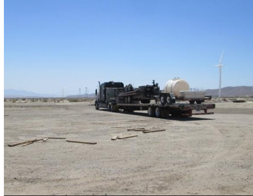
Photo 2: Construction crews continue to remove construction equipment and materials from the laydown yard.
