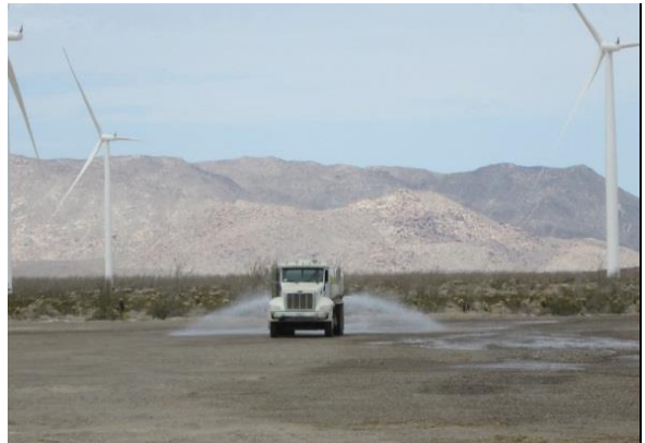
Photo 4: Construction crews utilize water to minimize dust emissions during removal of construction equipment and materials at the laydown yard in accordance with the Dust Control Plan (MM-Air-1).
