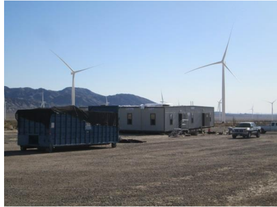
Photo 2: Construction crews were observed removing construction trailers from the lay down yard during this reporting period.
