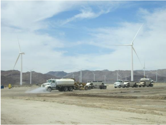
Photo 1: Gravel that was utilized to stabilize disturbed areas of the laydown yard was observed being removed from the right-of-way during this reporting period.
