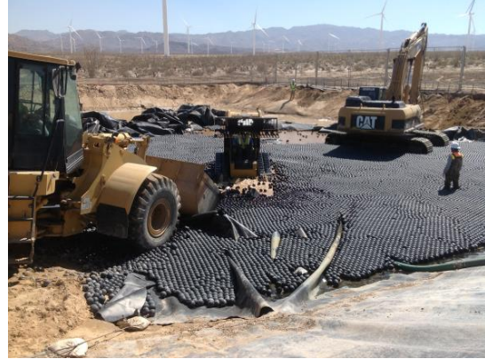
Photo 2: Construction crews began to remove the temporary water pond during this reporting period.
