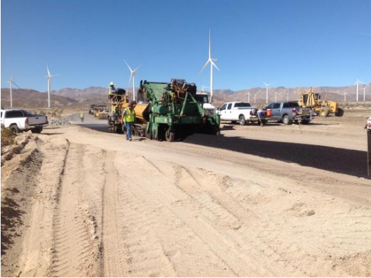
Photo 1: Construction activities associated with paving Dos Cabezas Road continued during this reporting period.
