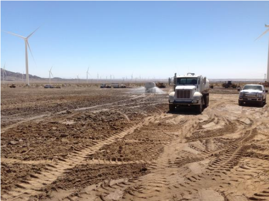
Photo 3: Construction crews utilize water to minimize dust emissions in accordance with the Dust Control Plan (MM-Air-1).
