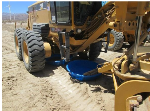
Photo 4: Construction crews place containment basins beneath construction equipment staged at the laydown yard in accordance with MM-Water-9 and MM-Water-10.
