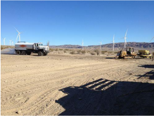
Photo 1: A water truck is utilized during revegetation activities at the Laydown Yard in accordance with MM-AIR-1 and the Dust Control Plan.
