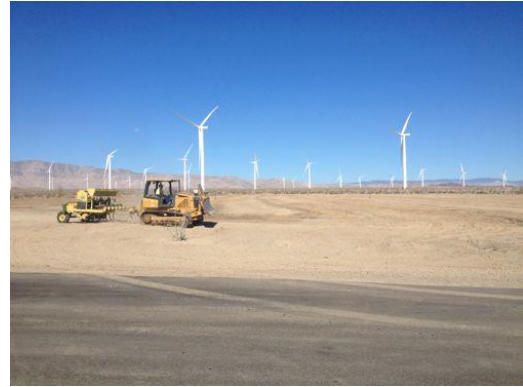
Photo 2: The BLM approved revegetation specialist completes seed installation via use of an imprinting machine at the Laydown Yard in accordance with Section 4.5.8 of the Habitat Revegetation Plan (MM-Veg-2b).
