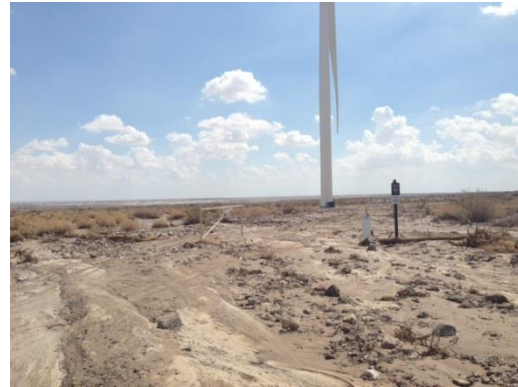
Photo 4: Wind Turbine Pad Site #128 following the rain event on July 21, 2013. OE LLC is anticipated to complete repair of access roads and BMP's during the next reporting period.
