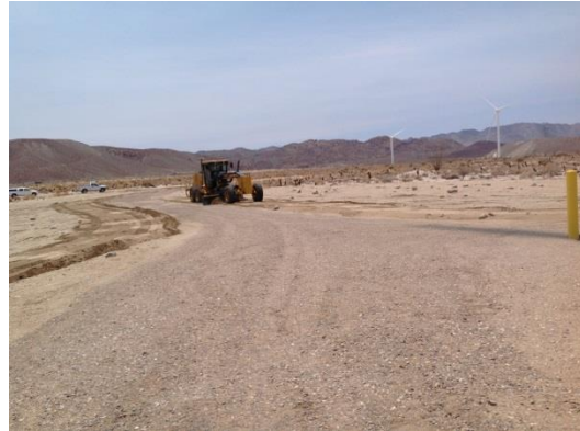
Photo 2: A belly scraper preparing the work area for blade replacement activities. All construction activities were completed within the approved work limits during this reporting period.
