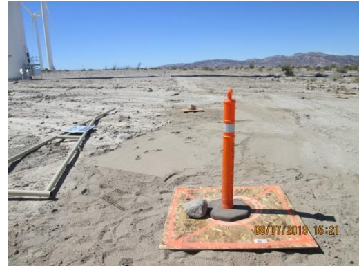
Photo 4: Construction crews place plywood over excavations at the completion of daily construction activities to prevent wildlife entry (MM-WILD-1B).
