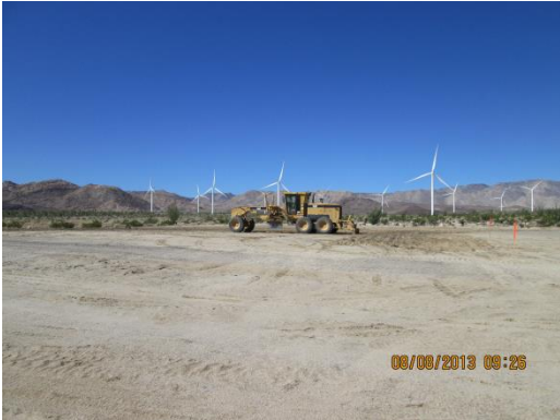
Photo 1: Construction crews established crane pad sites and wind turbine blade staging areas for blade replacement activities during this reporting period.
