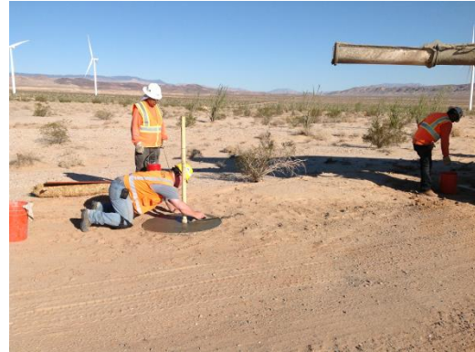
Photo 2: Crews reinforce access control gates located at the entrances to wind turbine pad sites. The access control gates are required in accordance with the Access Control Plan approved by the BLM (MM-CUL-11).
