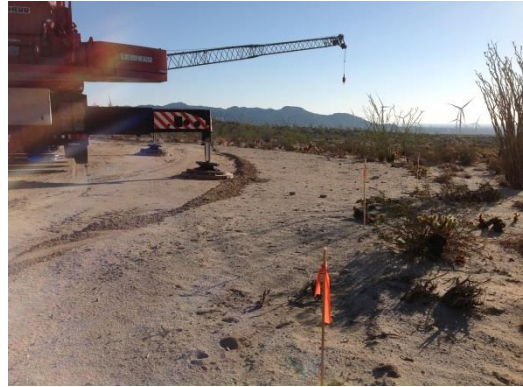
Photo 6: Construction crews place survey stakes to identify the approved work limits prior to ground disturbing activities (MM-VEG-1A).
