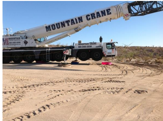
Photo 8: Containment bins are placed beneath construction equipment to minimize the potential for equipment fluids to be discharged onto the ground in accordance with the SWPPP (MM-HYD-9).
