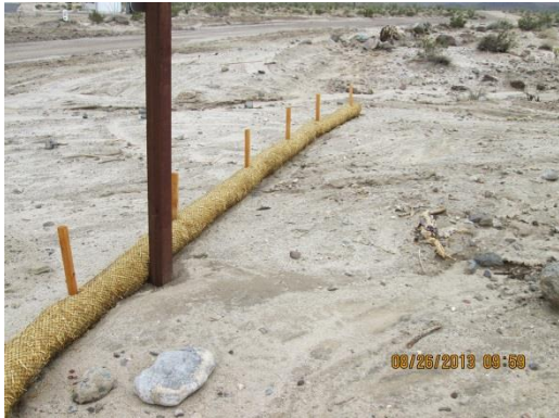
Photo 3: Installed straw wattles required as a best management practice in the SWPPP (MM-WATER 9) along a BLM-designated route of travel were observed to be in good working condition.
