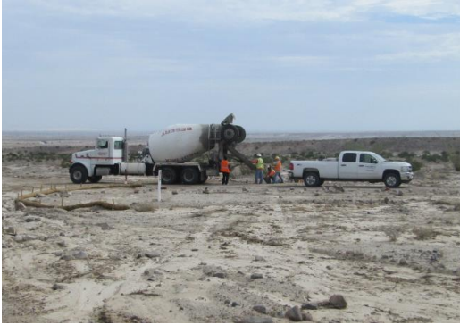
Photo 1: Crews reinforce access control gates located at the entrances to wind turbine pad sites. The access control gates are required in accordance with the Access Control Plan approved by the BLM (MM-CUL-11).
