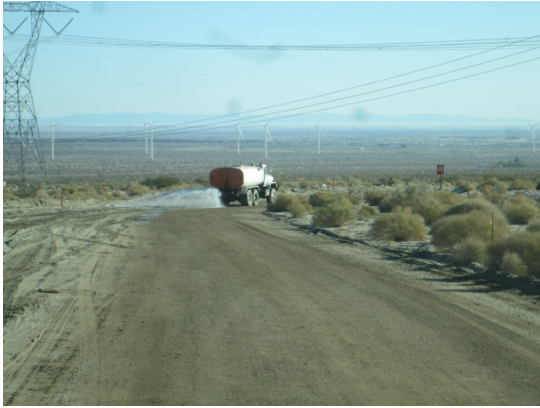
Photo 5: ECMs observed water trucks suppressing dust along turbine access roads in accordance with MM-Air-1.
