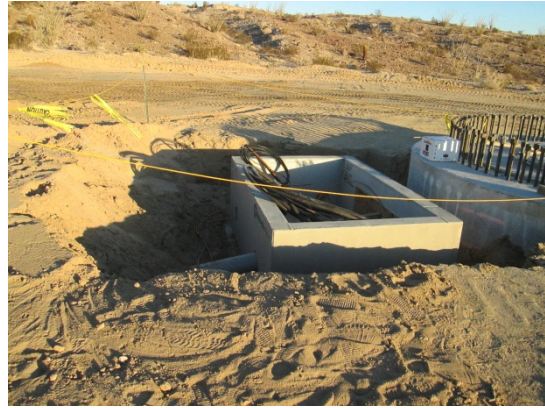
Photo 6: An excavation area adjacent to a wind turbine base foundation has sloped edges in accordance with MM-Wild-1m. Sloped edges in excavation areas provide wildlife with an escape ramp to prevent entrapment.
