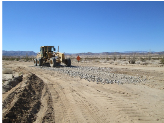
Photo 4: ECMs observed repair of a rock apron at an access road to a turbine site. The rock apron was noted as needing repair the previous reporting period.
