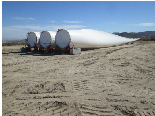
Photo 8: ECM's observed turbine part deliveries and staging within the approved work limits.
