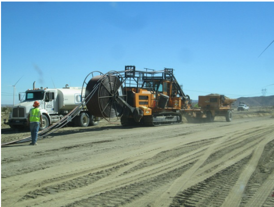
Photo 1: ECMs observed crews conducting non- initial disturbance sub-grade disturbance along turbine collection line trenching areas.
