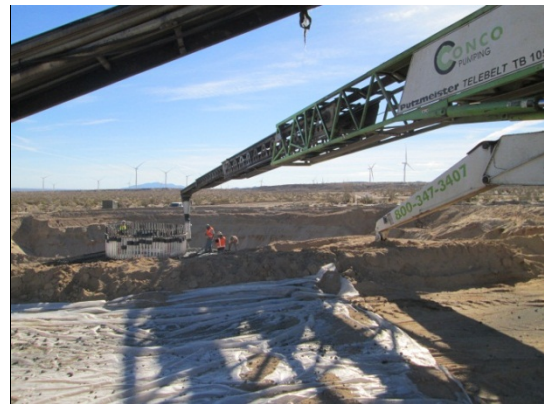
Photo 4: A concrete base pour is completed at a wind turbine foundation using plastic sheets placed along the ground surface to prevent soil contamination per the Storm Water Pollution Prevention Plan and Mitigation Measure Water-10.
