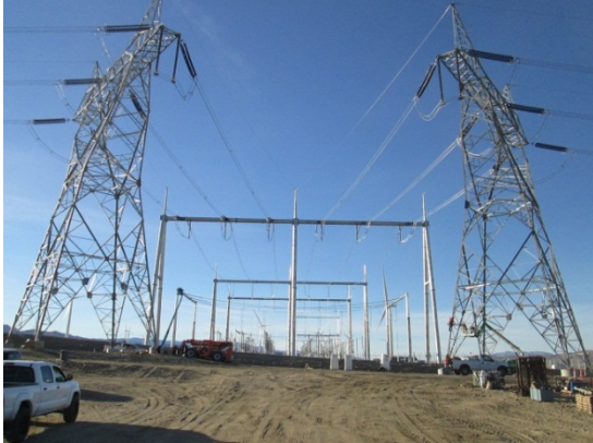
Photo 1: Testing and commissioning of the wind turbines and Substation/Switchyard began during this reporting period.
