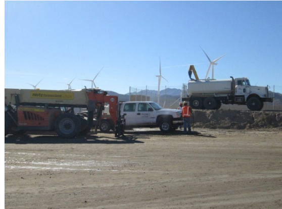
Photo 2: Construction vehicles are washed at the temporary laydown yard in order to minimize the potential for invasive species in accordance with MM Veg-1d and the Integrated Weed Management Plan.
