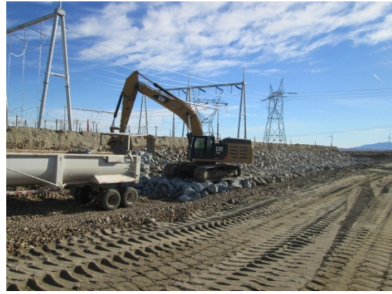
Photo 6: Environmental Compliance Monitors observed crews installing rip-rap around the substation switchyard for flood protection.
