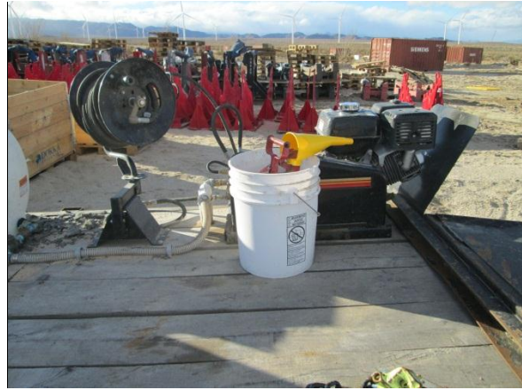
Photo 2: A gas container is placed within a secondary containment bucket to prevent soil contamination per the SWPPP and Mitigation Measure Water-10.
