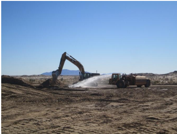
Photo 3: ECMs observed continued foundation excavation in preparation for wind tower foundation installation. Water continues to be applied in accordance with MM-Air 1 to control fugitive dust
