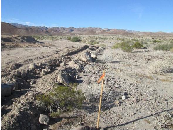
Photo 1: ECM's continued to observe delineation of approved disturbance areas/work areas within the right of way and flagging remaining intact.
