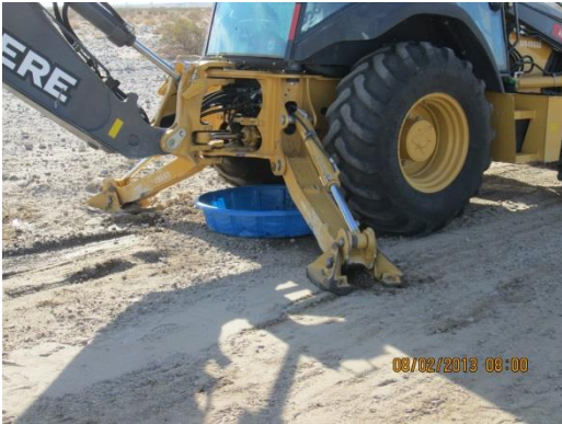
Photo 3: Containment bins are placed beneath construction equipment to minimize the potential for equipment fluids to be discharged onto the ground in accordance with the SWPPP (MM-HYD-9).
