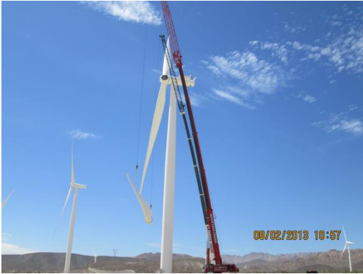
Photo 1: Construction crews utilize cranes to replace a wind turbine blade at Wind Turbine #90. All construction activities were completed within the approved work limits.
